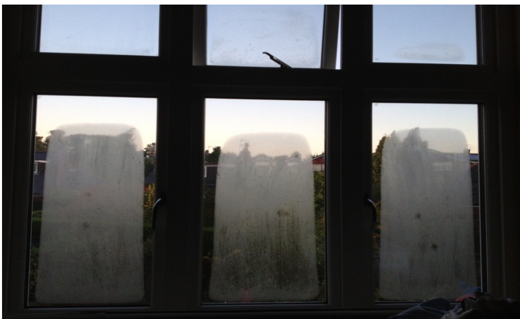
fig 1 – External condensation , border effect and pad residue on A Rated EnergiMAX™ DGU installation
